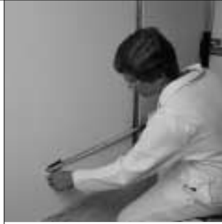
20. Reference locations such as floor surface or panel edges are very helpful.
