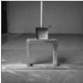
4. A saddle can also be fabricated from strut runner for electrical box support.
