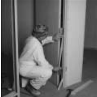
8. Sections of mortised trim are cut and snapped in place to fill above and below all hinges.
