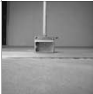
5. In some areas electrical boxes can be located in the floor track.
